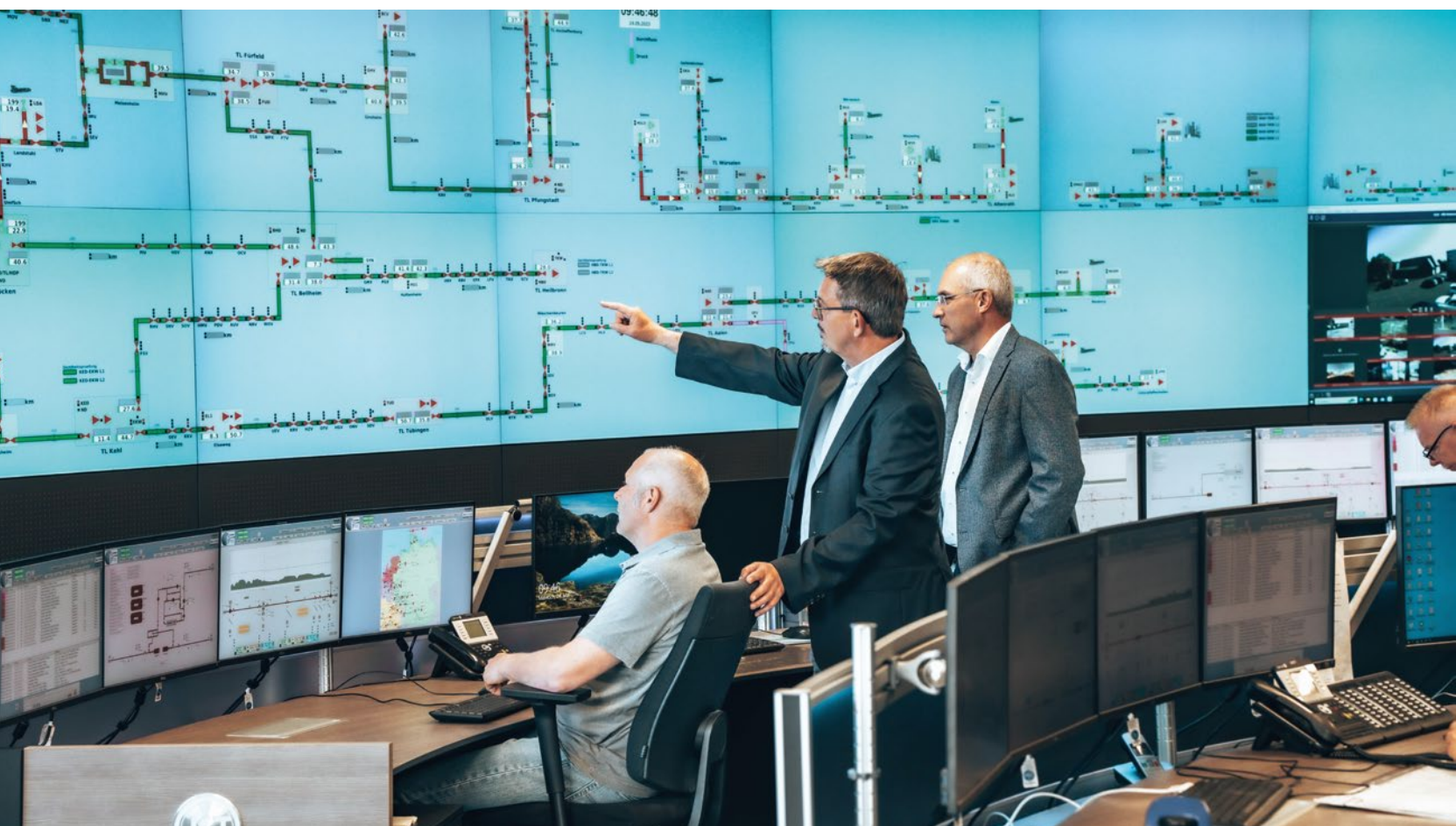
Control room for 24/7 monitoring of all pipelines
