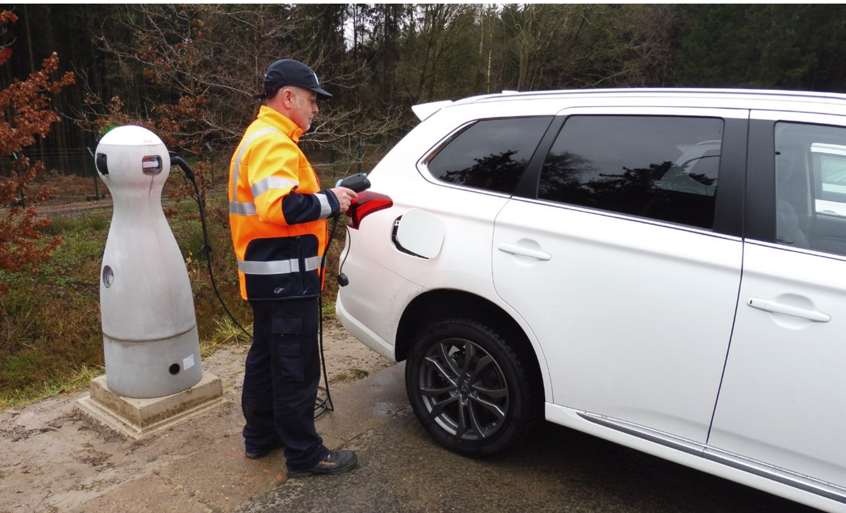
Electric vehicle charging station in a depot
